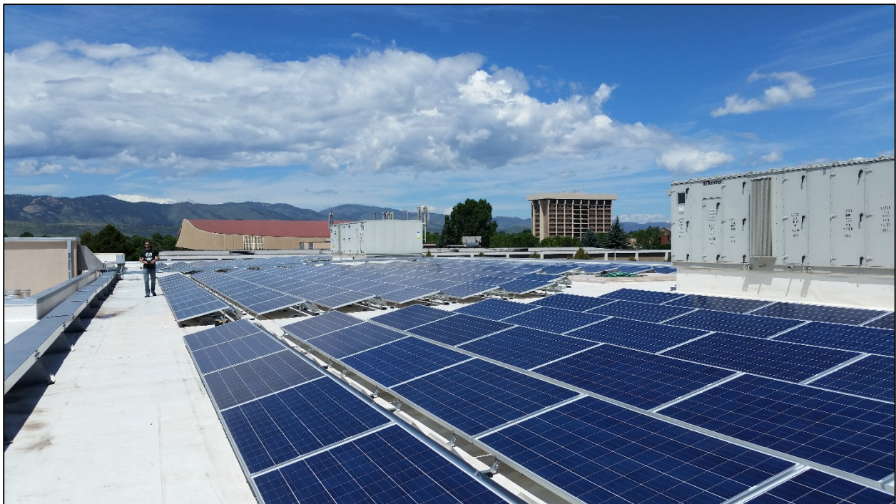
545 kW solar array located on the Student Recreation Center at CSU
