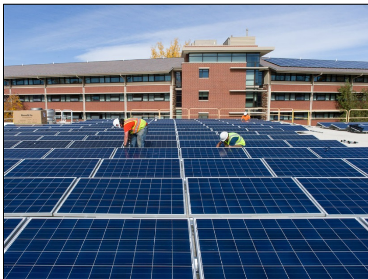
Solar array installed on Braiden Hall as part of the City of Fort Collins SP3 Solar Power Purchase Program
